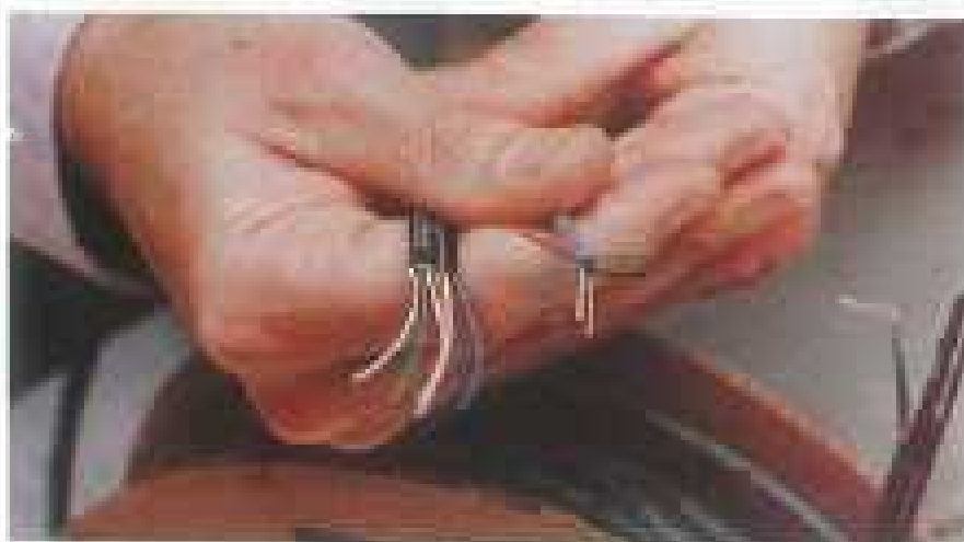
A new type of telephone cable is being installed by the Post Office. Undercarpet cable is flat and designed to be laid on the floor and covered by carpet. Carpet tiles are the preferred covering as they allow easy access when the Post Office needs to make repairs or alterations.
